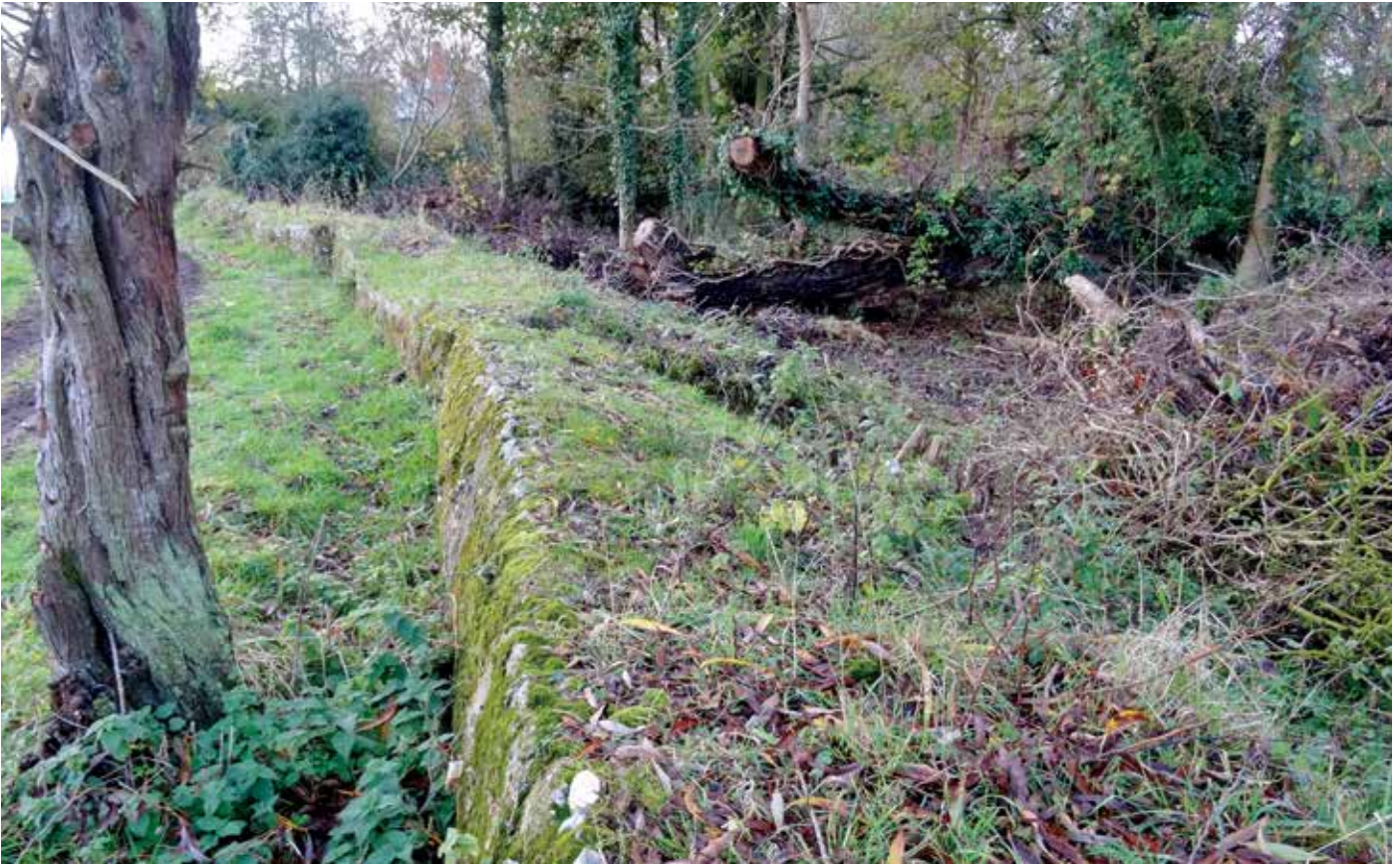
Fig 5: Burnham Norton. Natural soft capping of north wall.
