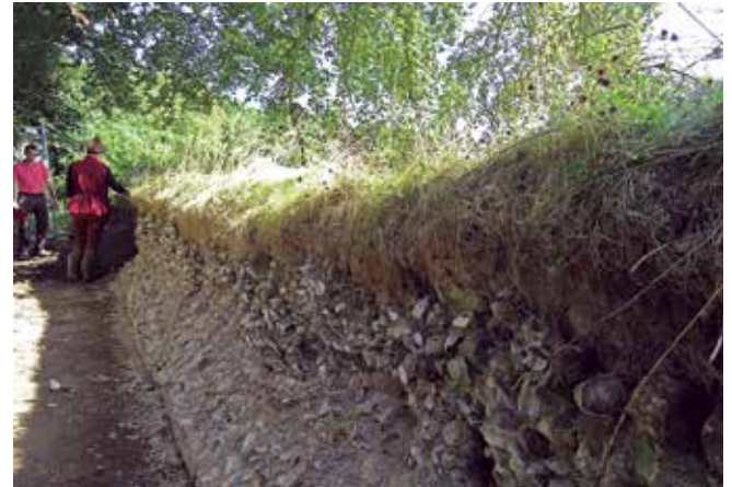
Soft-capping on the precinct wall. Research carried out by English Heritage has found that soft capping can provide effective protection from thermal fluctuations and freeze-thaw action.
